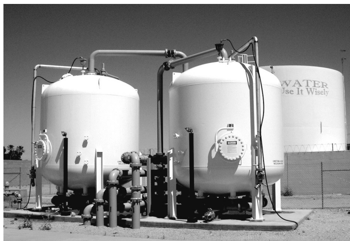
Pictured above is the South Shannon Water Treatment facility. As of March 27, 2012, approximately 22 million gallons of water has been treated since the seveneenth carbon change-out on February 22, 2012. A total of 1.1 billion gallons of water has been treated by the treatment system since its start up in July 2006.
