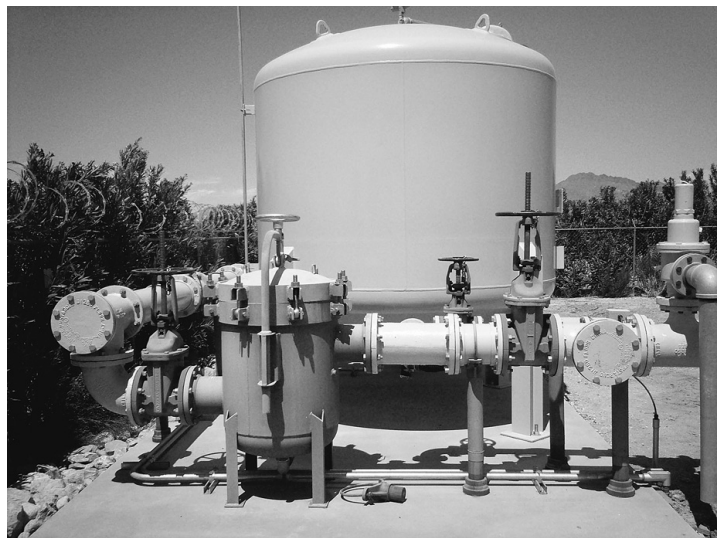
Pictured above is the Diablo Village Well No. 1 Arsenic Treatment System, installed in 2011 at a cost of $252,000
