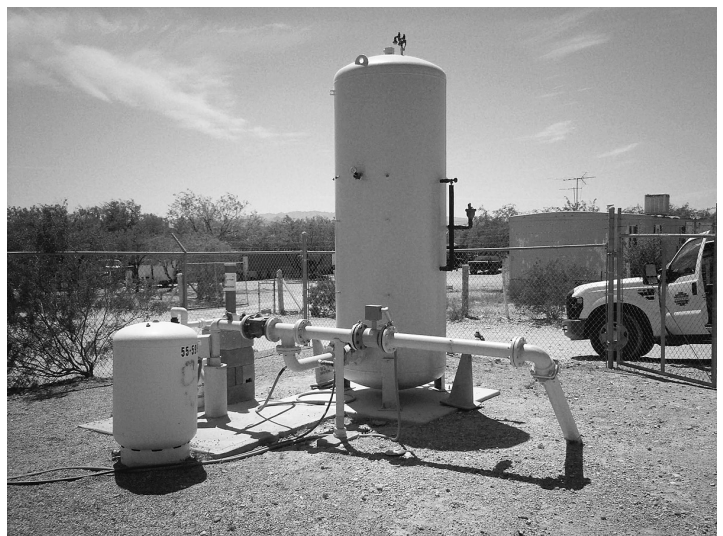
The above photo is of the Metro Southwest E&T Well No. 23. This well provides water service to many of the customers within the E&T area. The photo depicts the well, chlorination, and the surge tanks to help maintain the system pressure. Six months ago District staff replaced the smaller surge tank (on the left) with a 1,000 gallon surge tank to provide for less cycling of the well and the ability to maintain better system pressure
