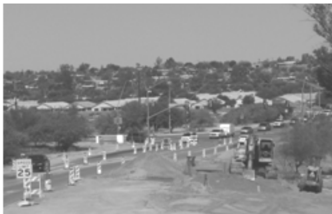
Motorists must deal with traffic control while waterline construction precedes the actual road construction.
