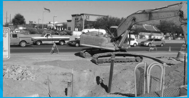
Construction at Oracle Road and Magee Road intersection, one of last RTA project areas to be addressed by Metro
